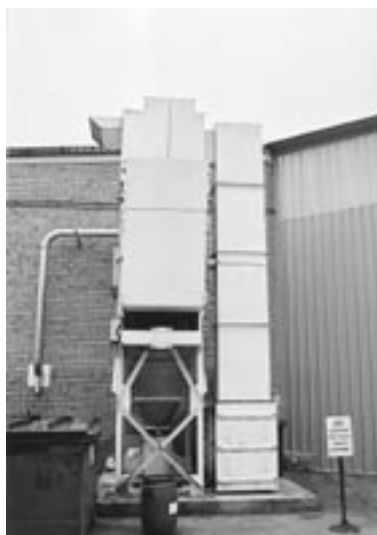
An APCD used for dust extraction and collection which vents through an appropriately configured stack (stack not visible).
