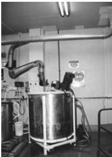
Engineering controls such as local exhaust ventilation and extraction of dust and odours helps protect the environment and personnel health.
