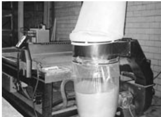
A baghouse filter fitted to a local exhaust ventilation and extraction system on a piece of woodworking machinery. The bottom fabric bag has been replaced by a thick durable plastic bag which aids the cleaning process, reducing dust and particulate emissions.
