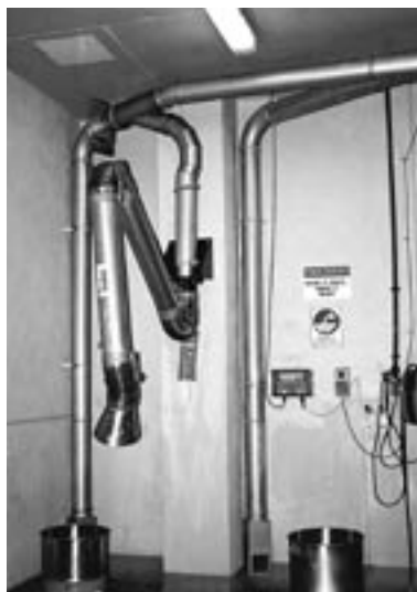
Local exhaust ventilation should be used to remove fumes and dust produced by the welding process.
